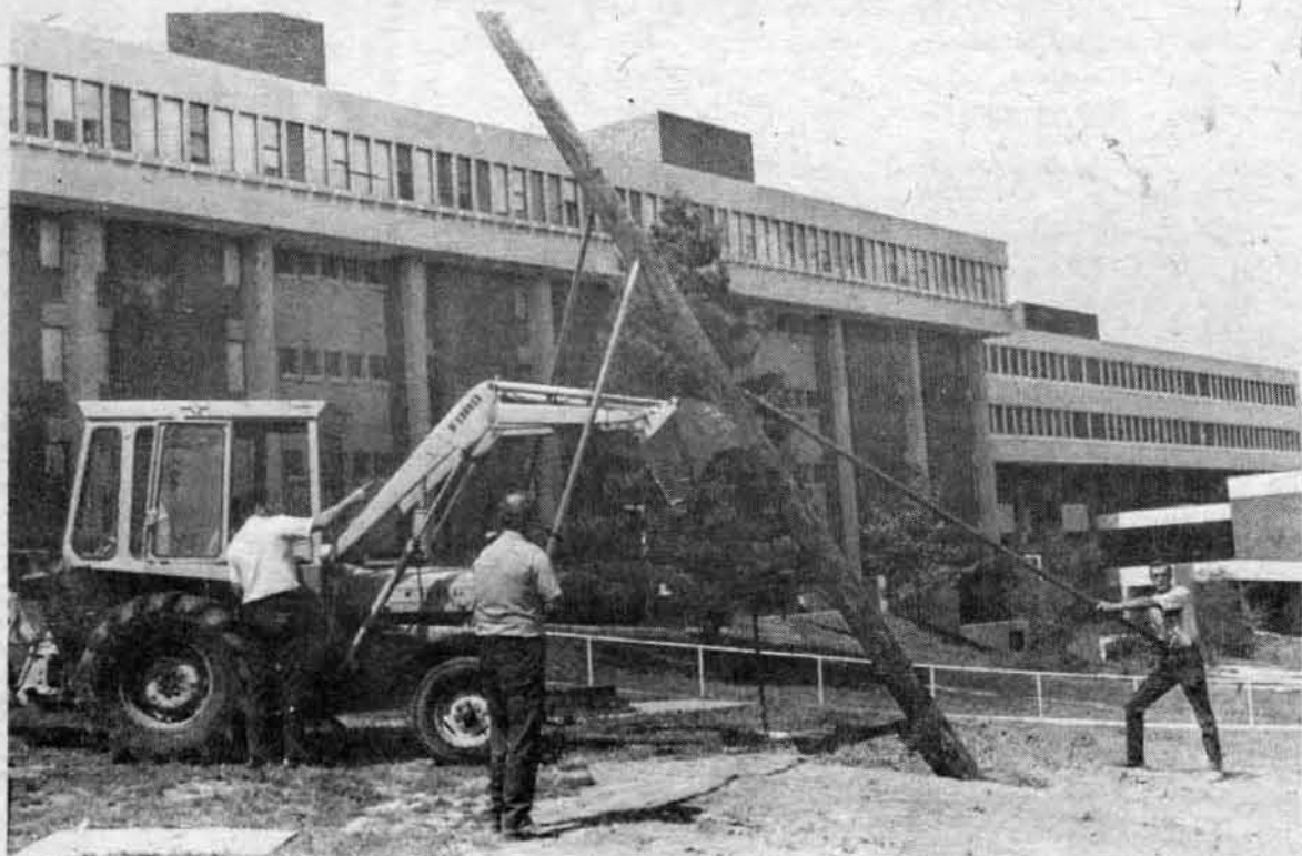
PULL: Workmen put the finishing touches on the asphalt area by Clark Hall. The pole will hold the lighting facilities for night use of the volleyball/basketball court [photo by Romondo Davis].
